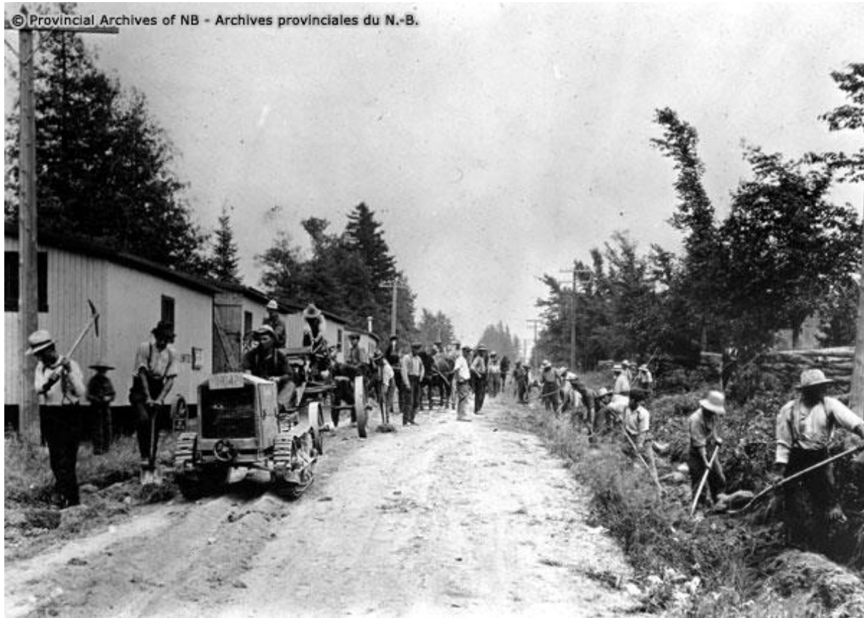
Men and machinery work together to build a road at Shogomoc, a former community between Nackawic and Hawkshaw.
